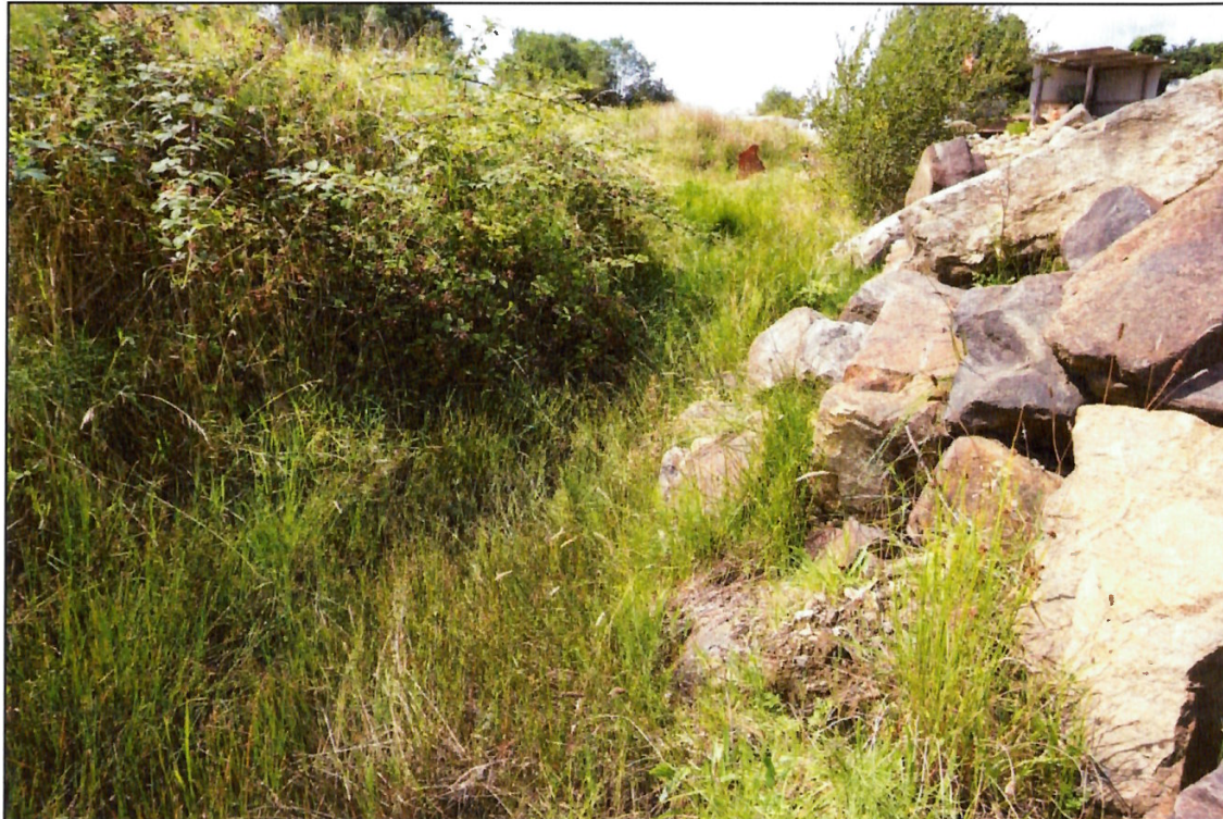
Photograph 4.5: The impeded pathway from the outflow of the main settlement pond to the discharge point.
